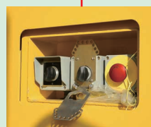
Engine room front
